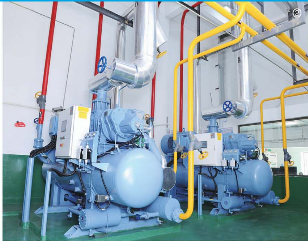
Picture ①: Big scale brine tank type ice making system
